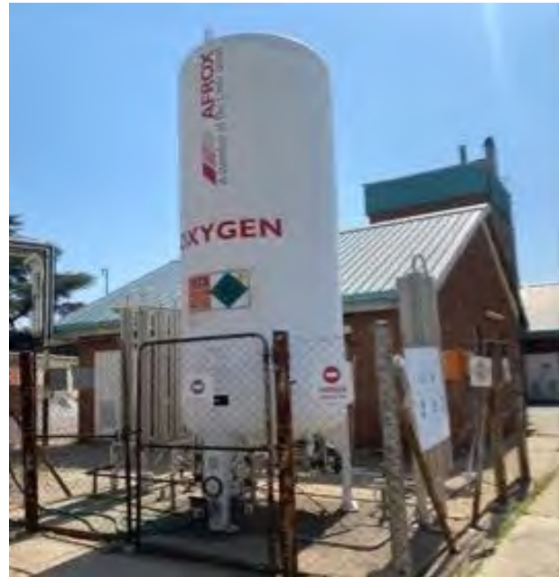
A 15-ton Afrox supplied liquid oxygen tank at a hospital
