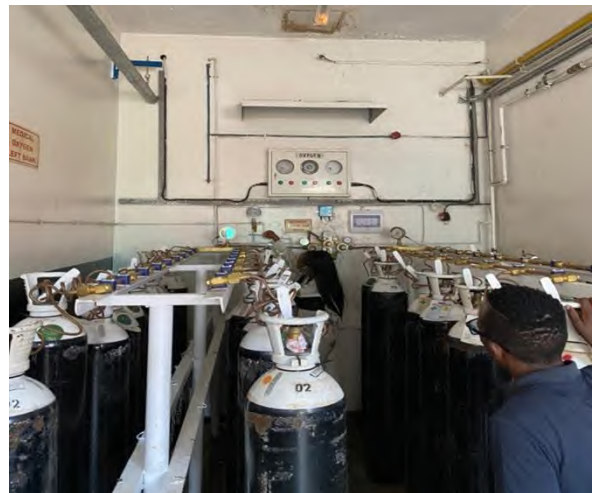
Hospital oxygen bank connected to a manifold
